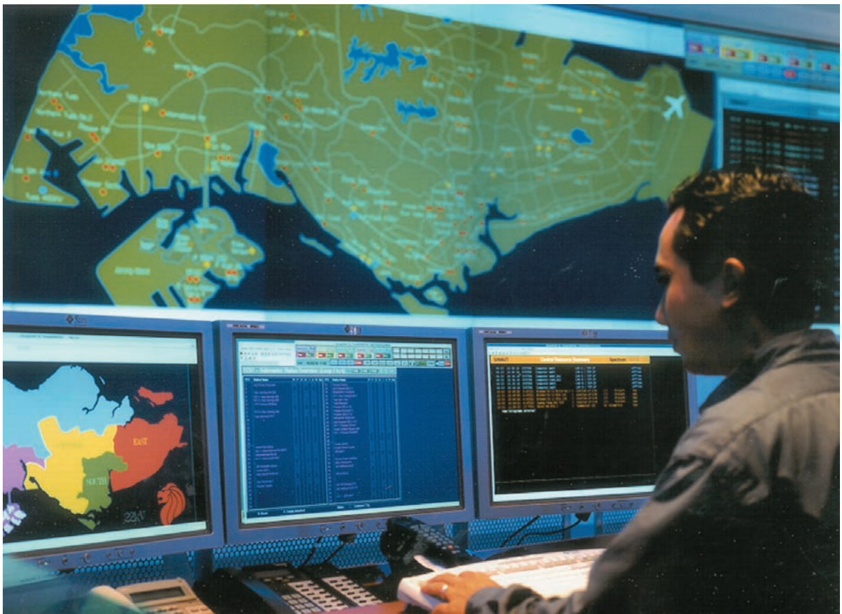
24-hour Monitoring via SCADA System
